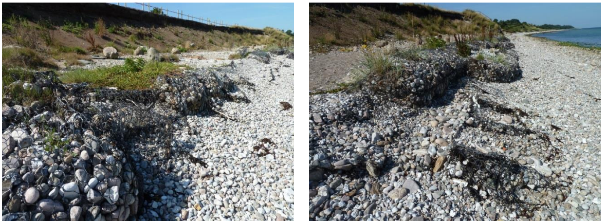
Figure 17.9 Damaged Gabion revetment at Lumsås, Denmark. Damages occurred during the extreme storm "Bodil" on 6 th December 2013.
