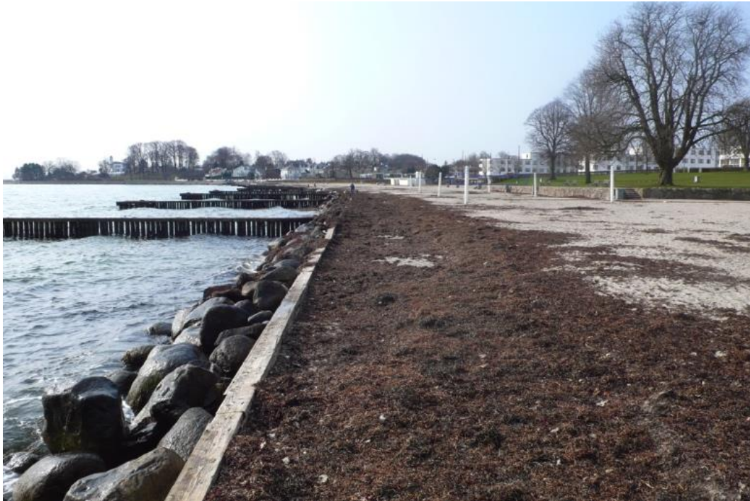
Figure 17.12 Small wooden wall supported by stone revetment in front, and piled groynes protecting artificial beach at Bellevue, Denmark. (Constructed in the 1930ties but now replaced by a natural beach).
