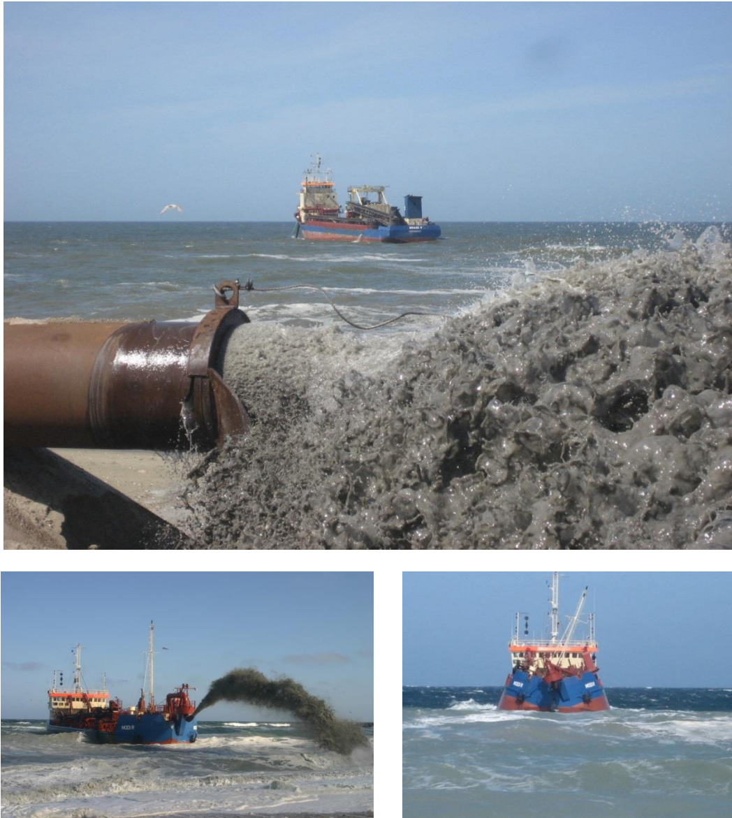
Figure 17.50 Nourishment methods in practice by the Danish Coastal Authority. Upper: Beach nourishment by pipe discharge on the beach. Lower: Left: Foreshore nourishment by over the bow pumping and right: Shoreface nourishment by split barge. From: Rohde Nielsen.
