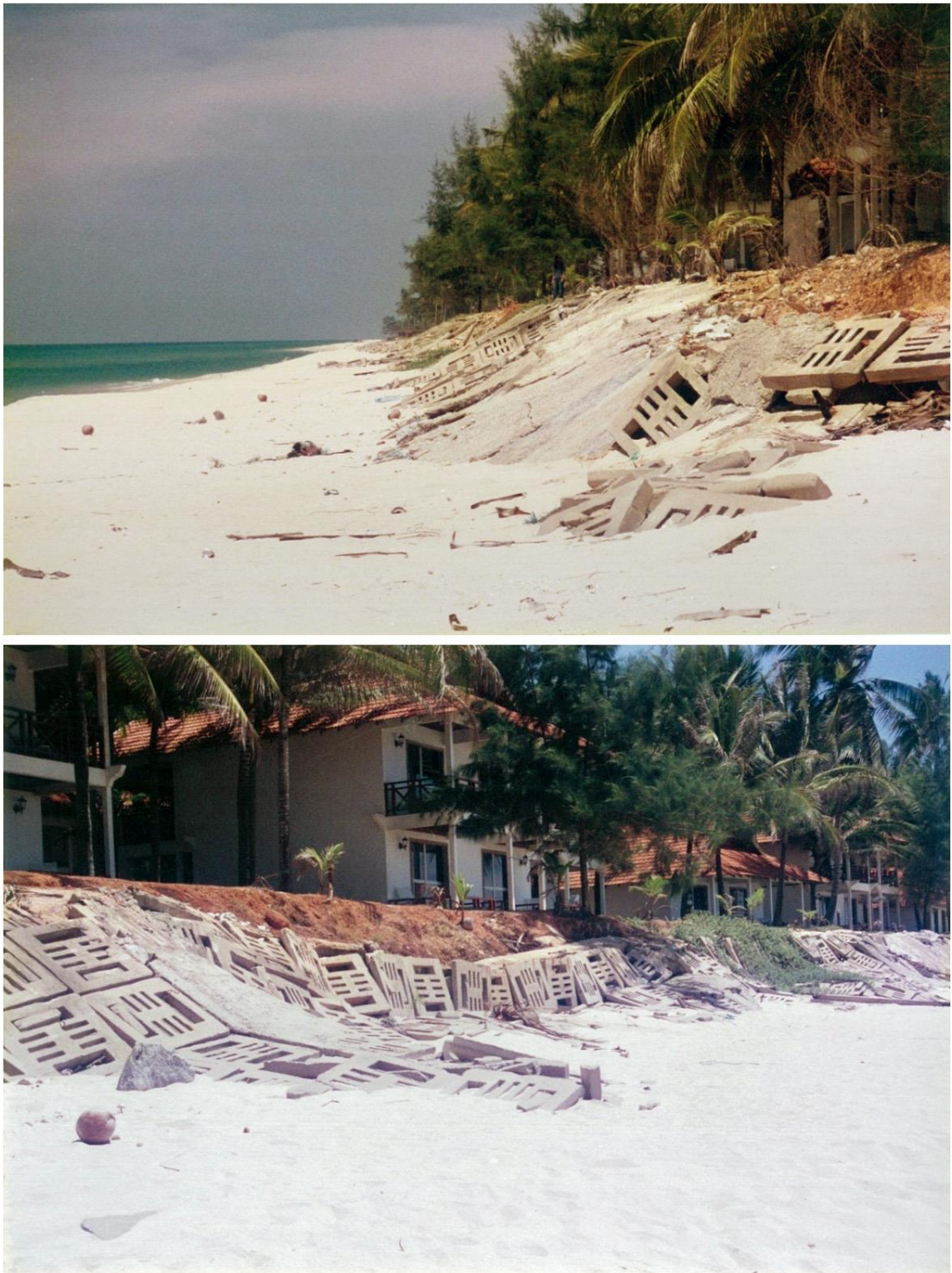
Figure 17.5 Damaged Flex Slab revetment south of Merang in Terengganu, Malaysia.
