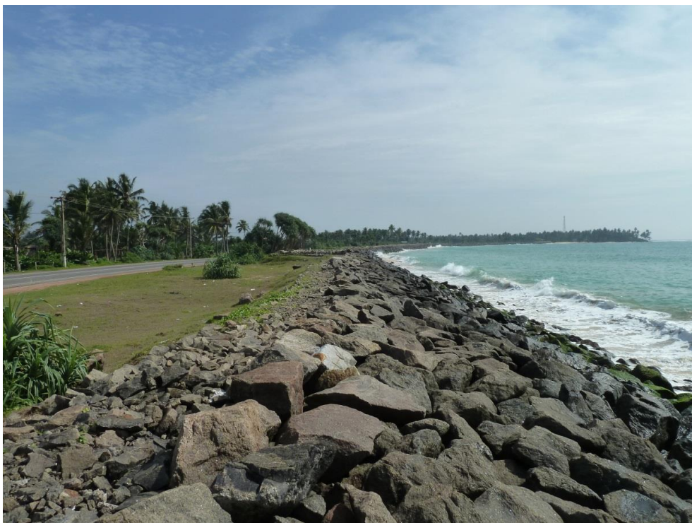
Figure 17.3 Rubble mound seawall protecting the coastal road at Madampagama, SW coast of Sri Lanka.
