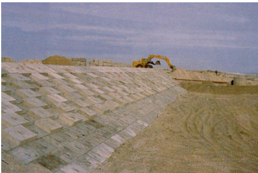
Figure 17.13 An example of a buried revetment constructed in concrete blocks, the revetment will later be buried into an artificial dune. (Danish Coastal Authority).
