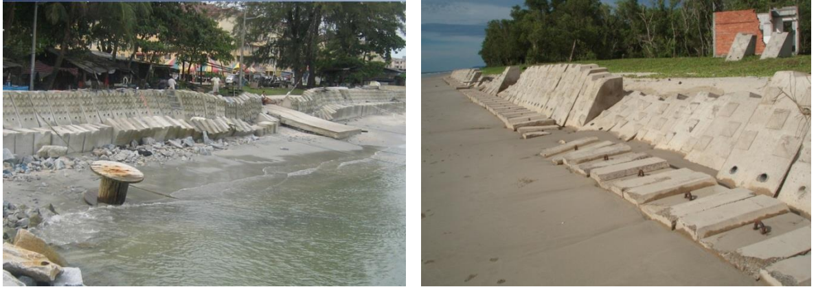
Figure 17.8 Examples on failures of concrete block revetments in Malaysia. Left: By scouring of the toe (Penang), Right: By overtopping (Labuan).
